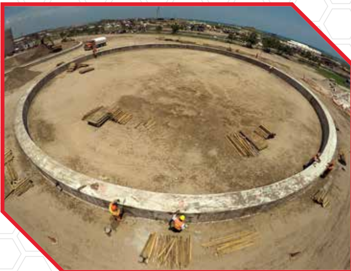
Foundation optimization to support a 26m diameter tank with a concrete reinforced foundation ring.
